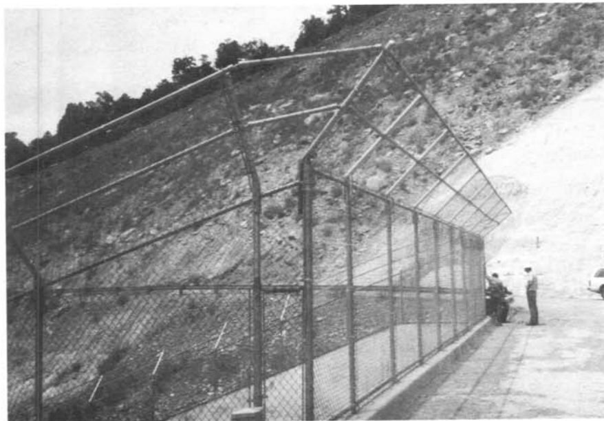
Spillway fence extension to prevent rocks from being thrown onto the chute floor.
