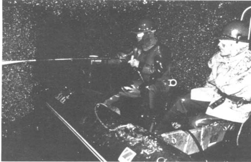
Photo 3.-Water at high pressure has been used to blow zebra mussels off walls of invested chambers at electric power stations, municipal waterworks, and pumping stations. Freed mussels must be collected to prevent them from washing downstream into screens, nozzles, and other constrictions when cleanup is over and plant operation resumes.
