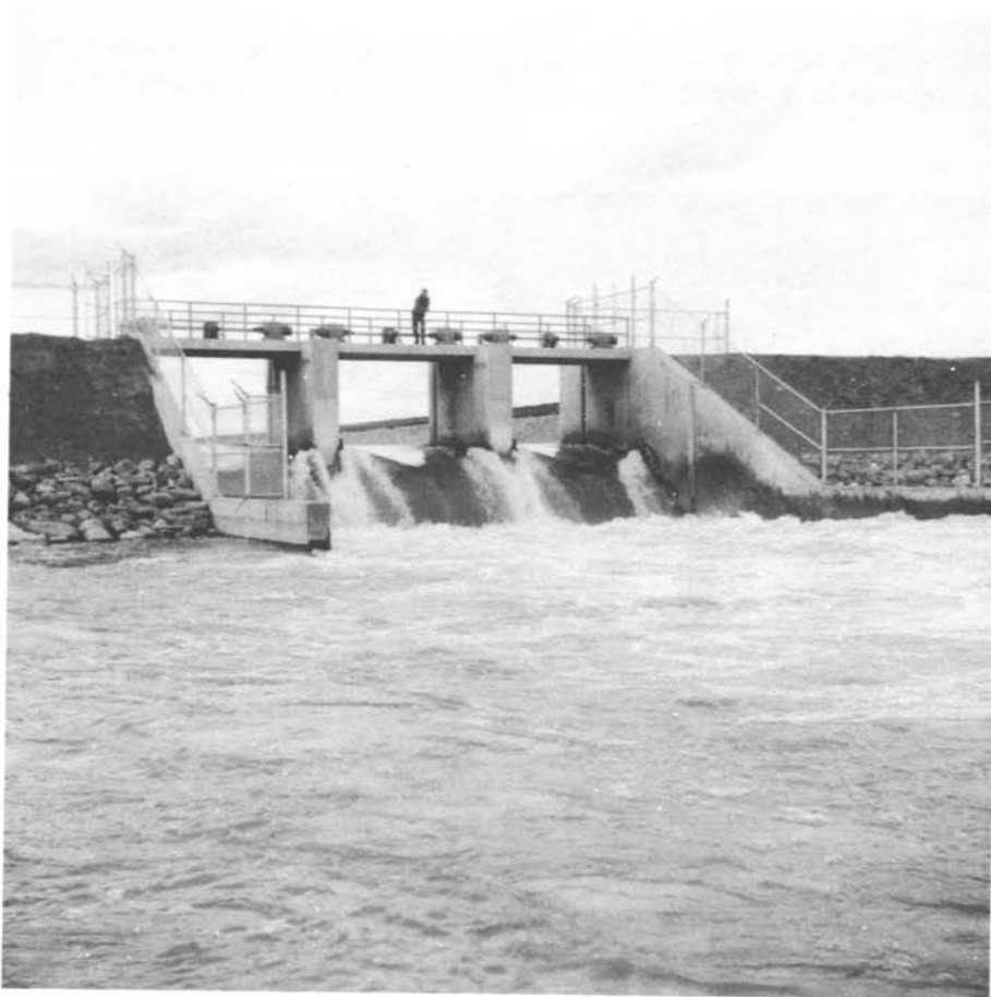
Drop No. 18 on the St. Mary Main Canal is a check drop structure with three Overshot Gates.
