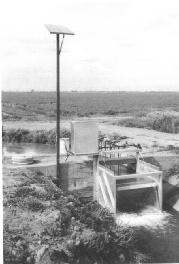
This smaller automated Overshot Gate is solar-powered, but these gates can also be connected to the local electrical grid system.
