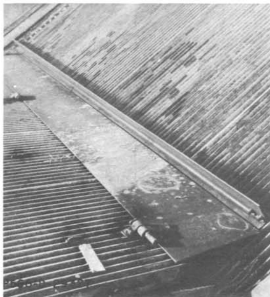
Flap Gate at Bottom of Canal Fig. 188C
