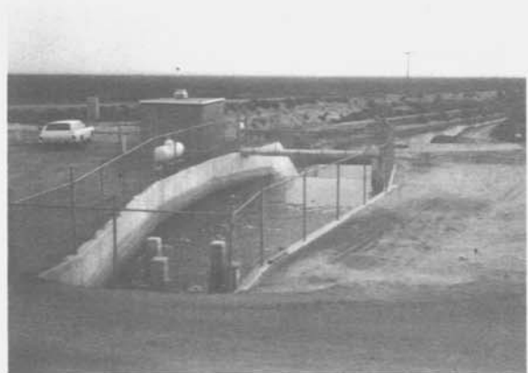
Figure 10.—Typical customer turnout site.
