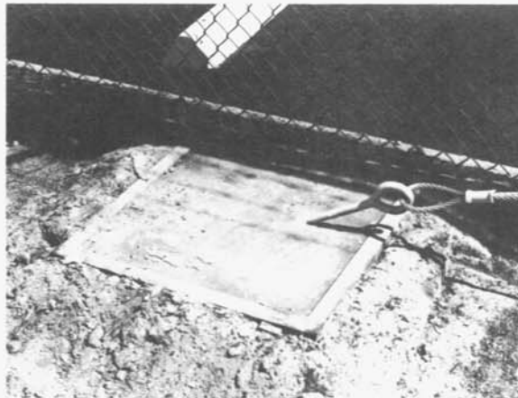
Figure 1.—Eye bolts set in concrete pads.
