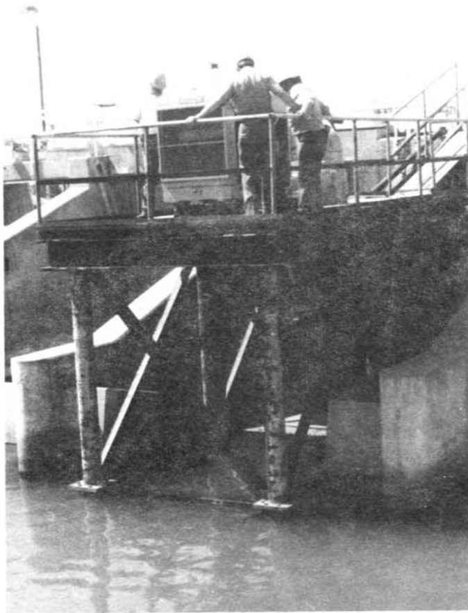
Figure 2. - View looking upstream at pump and platform installed between the gate arms at the Equalizing Reservoir check.
