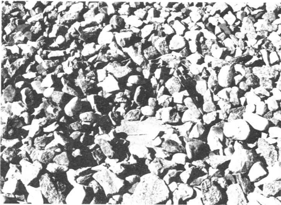
Figure 2. - Insufficient gravel cover exposing polystyrene foam on IRMA roof.
