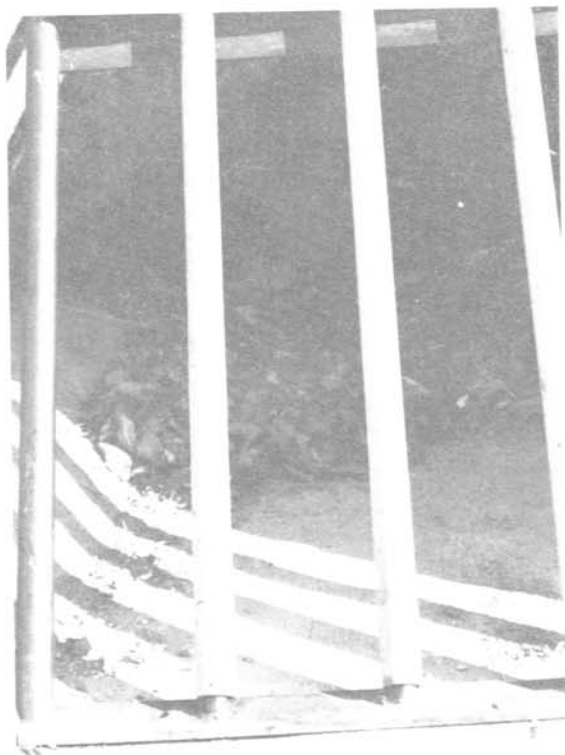
Figure 11 is a closeup view of the trashracks center section. Construction details of the removable pipe section, pipe pins, notch guides and frame are visible.
