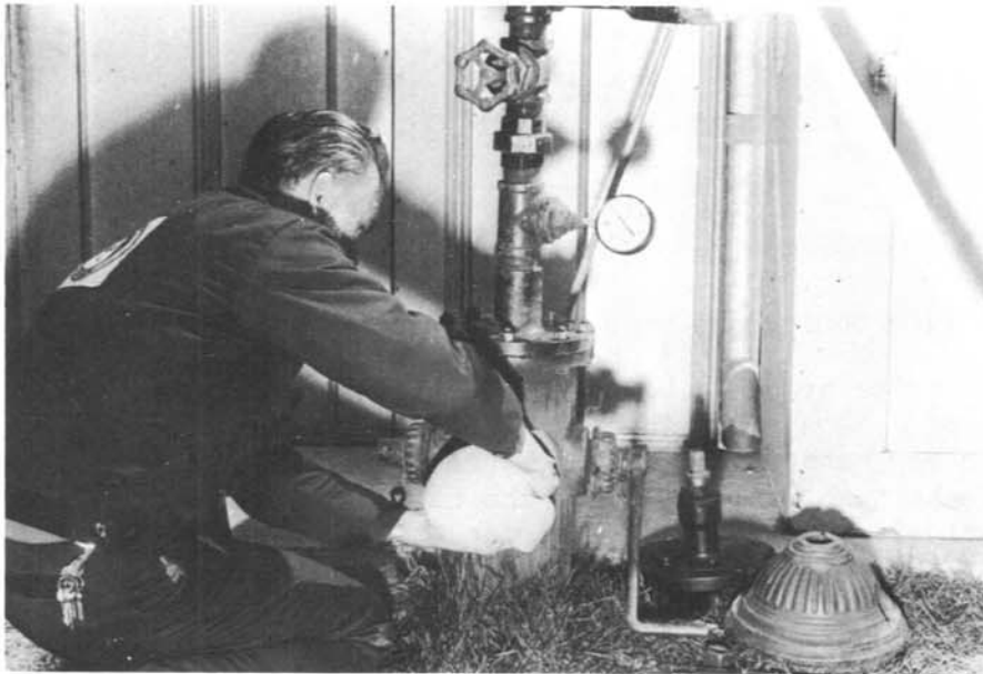
Figure 3. Hook-up for Propelling Swab Using Another Hydrant as Pressure Source. Photo P222-D-71333
