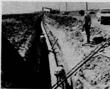
Installing concrete pipe on the San Luis Unit, Bureau of Reclamation's Central Valley Project, California. Photo P805-243-1176 NA
