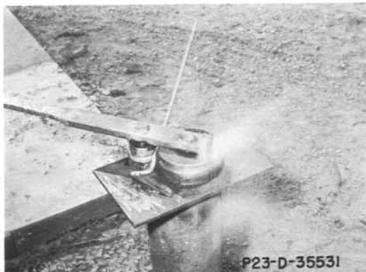
Fig. 3--Bender mounted on pipe support and initial position of re-bar before bending.
