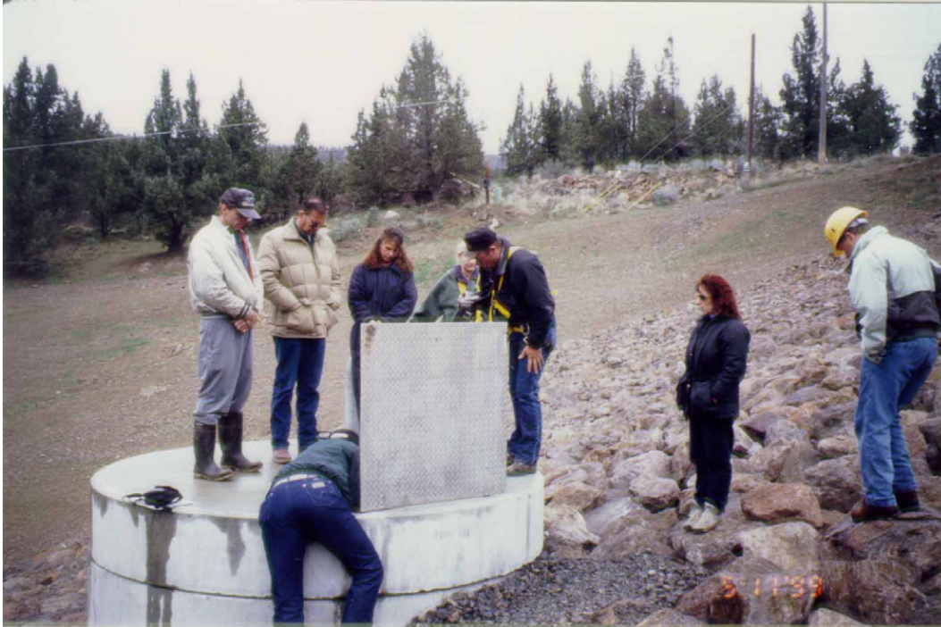
Figure 13.—Completed inspection well in the downstream face of a dam. Note that the upstream side of the inspection well is several feet higher than the slope. Also shown is a single leaf door for access. The individual to the right of the door is outfitted with a safety harness that connects to the safety rail on the ladder. This well installation utilized a safety rail along the ladder instead of intermittent landings along the ladder. This well is about 30 feet deep due to the overlying embankment fill.
