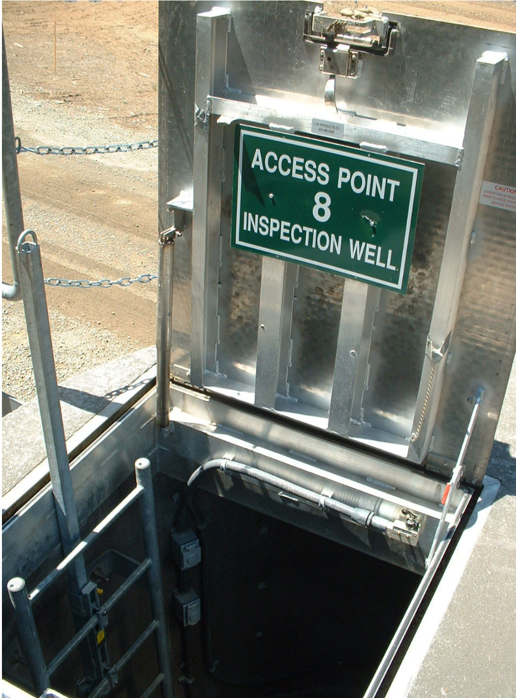
Figure 14.—Typical inspection well door, ladder, and grab bar. Also shown (right corner of door frame) is a switch that automatically turns on the ventilation when the door is opened. The grab bar is in the “up” position and is lowered in order to close the door. Also note the name of the well is on the inside of the door for protection. Nameplates posted on the exterior of the well are subject to vandalism.
