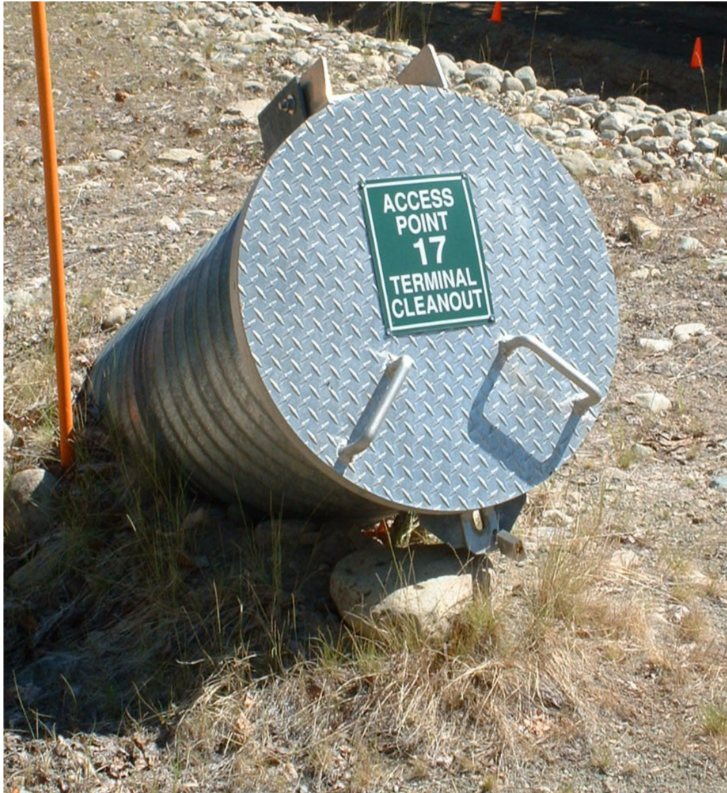
Figure 19.—Typical access point showing protective CMP pipe, lid, and lock.
