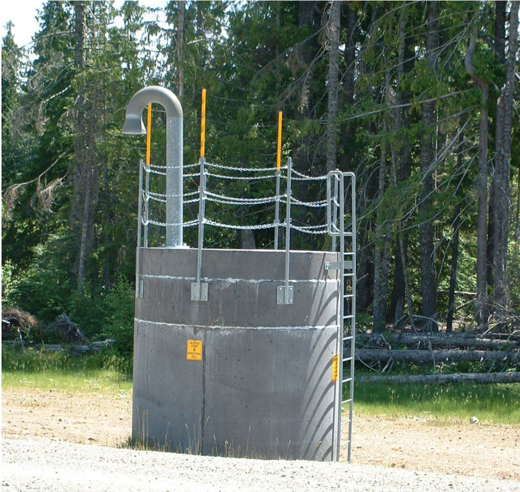
Figure 16.—View of the exterior of an inspection well. This well has a number of special features due to the local site conditions. The well was finished 10 feet above the ground surface due to the large amount of snow at this site. A ladder is provided on the outside of the well for access when snow is not present. A chain railing is provided on top of the well to prevent falls from the top of the structure. Three hazard markers were placed above the chain rail so snowmobiles would not hit the rail covered by snow. The well is also stained a dark gray to aid snowmelt on and around the structure. This well also has electrical power, active ventilation, and automated instrumentation.
