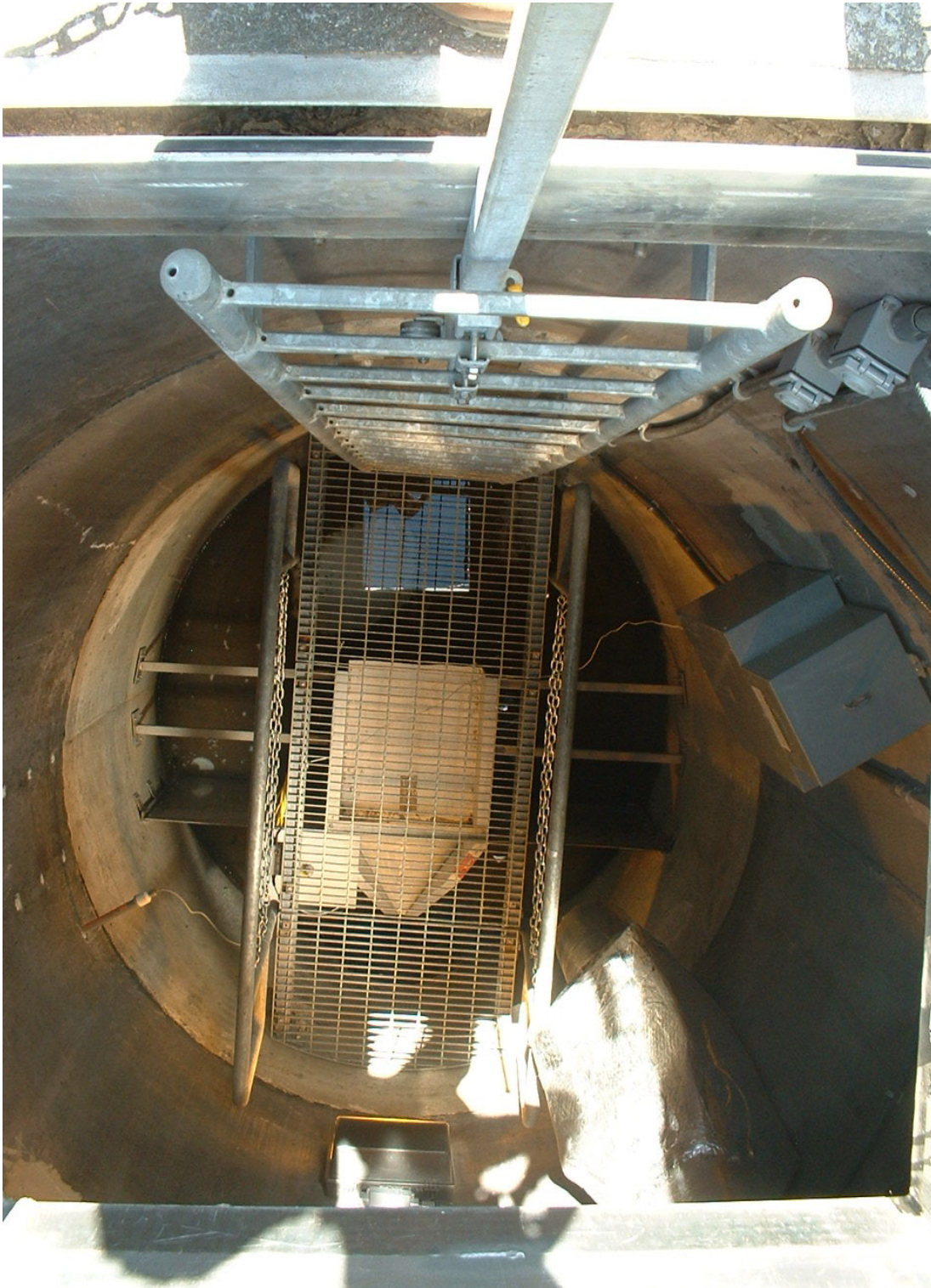
Figure 11.—View into a more sophisticated inspection well showing a landing for personnel and a flume. This well utilized aluminum brackets and a divider wall so the flume can be changed out.
