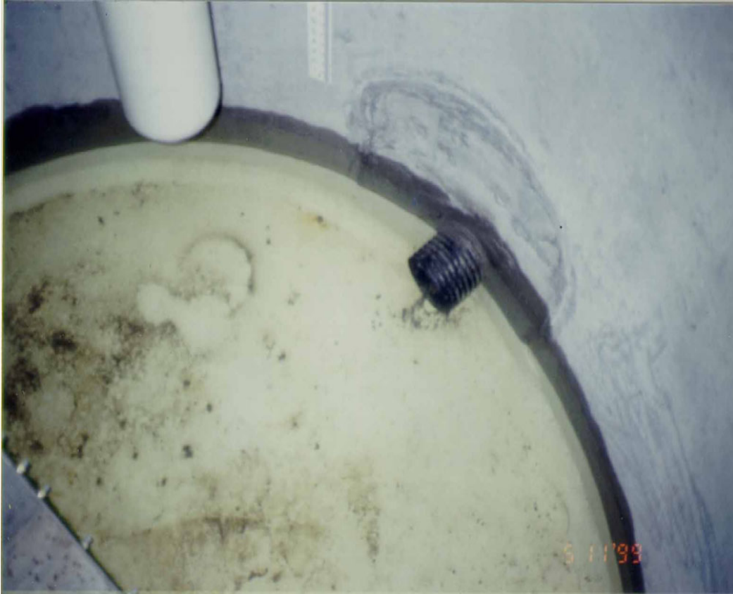
Figure 15.—View of a sediment trap in a typical inspection well. The bottom of the sediment trap is painted white so sediment is more easily detected. The photo shows a minor amount of sediment that discharged from the inlet pipe as well as material that fell out of the vent pipe shown in the upper left hand corner.
