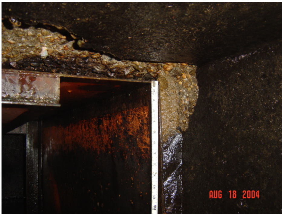
Concrete damage around steel liner (site visit).
