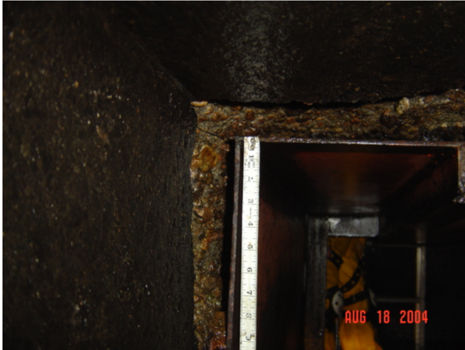
Concrete damage around steel liner (site visit).
