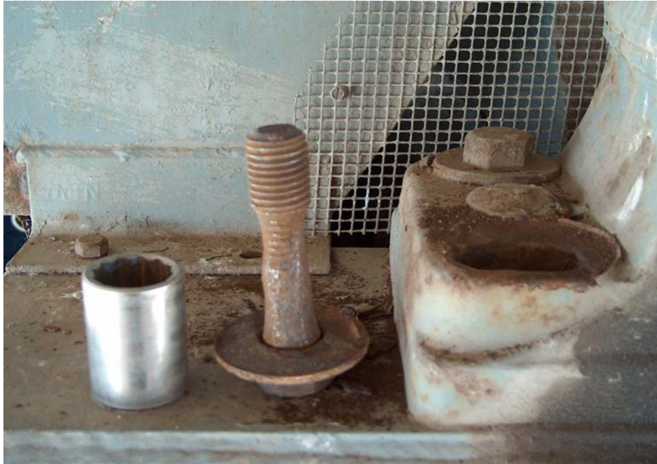
Photo 4.—Bearing bolt corrosion.
