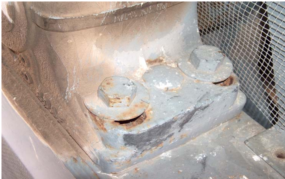
Photo 5.—Slotted holes not covered by washer.
