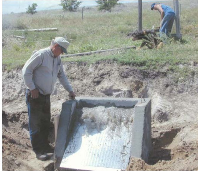
Figure 5.—Coanda-effect screen structure, similar to that shown in figure 4, operating at a relatively high flow rate. All flow still passes through the screen before reaching the toe.
