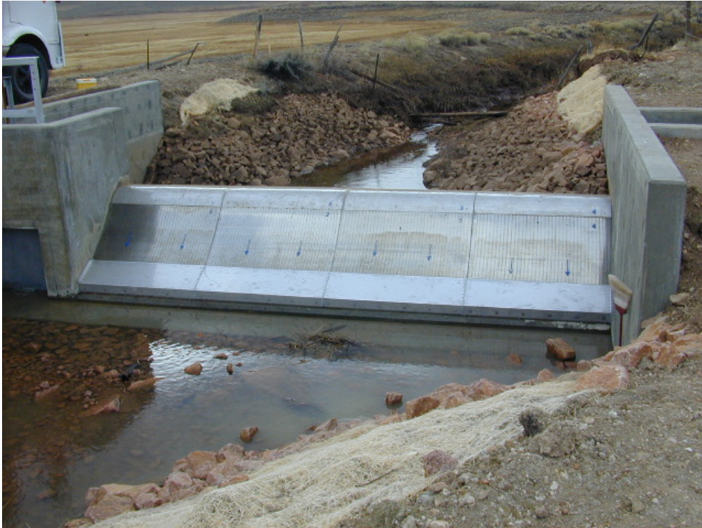
Figure 7.—Coanda-effect screen structure at Lake John, constructed in 2001. This structure replaced that shown in figure 6.
