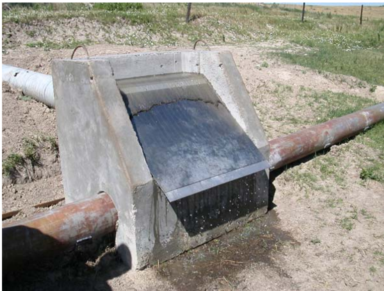
Figure 4.—Coanda-effect screen structure feeding two irrigation pipelines. Raw water enters the back of the structure through the white, polyvinyl chloride pipe. Screened water exits to the right and left. Overflow and debris are discharged onto the ground at the front of the screen.
