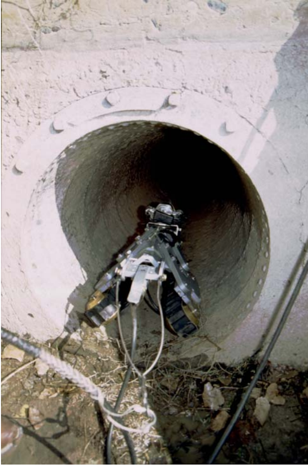
Photo 1.—Self-propelled inspection video camera entering a 24-inch-diameter siphon. Note the power cable and pull-out cable.
