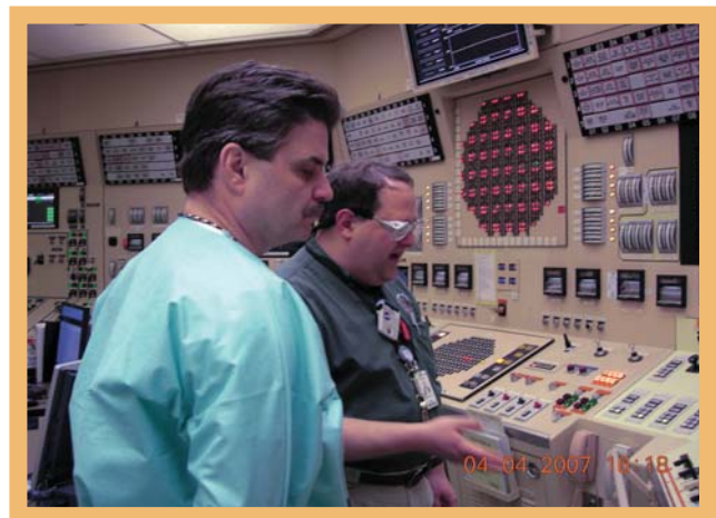
Senior Resident Inspector Dan Kimble showing the Region III Regional Administrator James Caldwell the condensate and feedwater control panel in the LaSalle Main Control Room.
