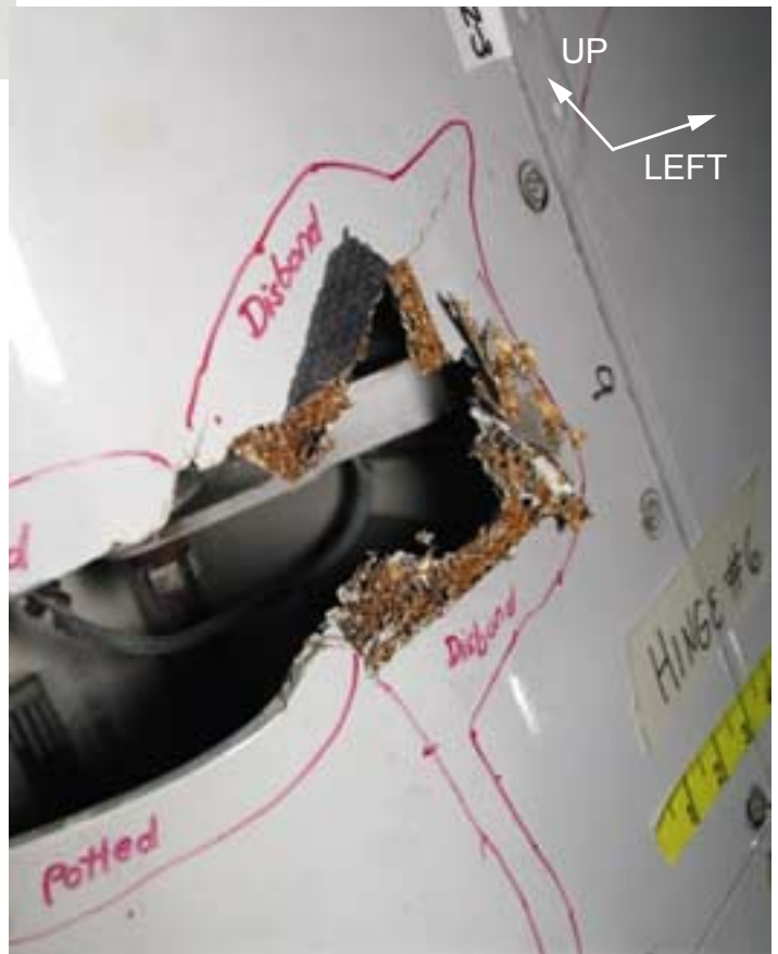
Figure 55. View of the left side of the LE fairing at hinge 6 showing damage to the left cutout end.
