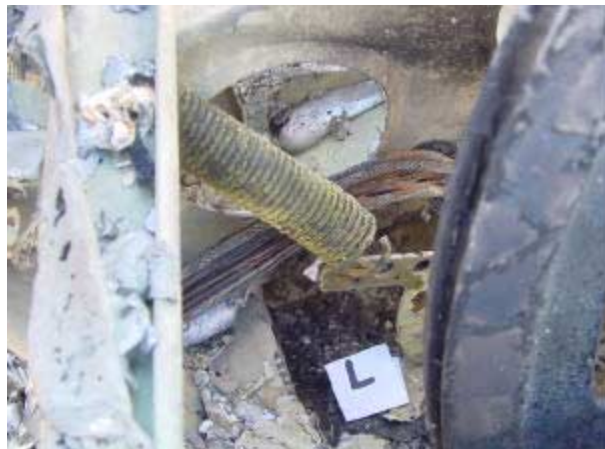
Photograph 8. Left spring as found attached to link. (Left edge of photo is toward nose of airplane.)
