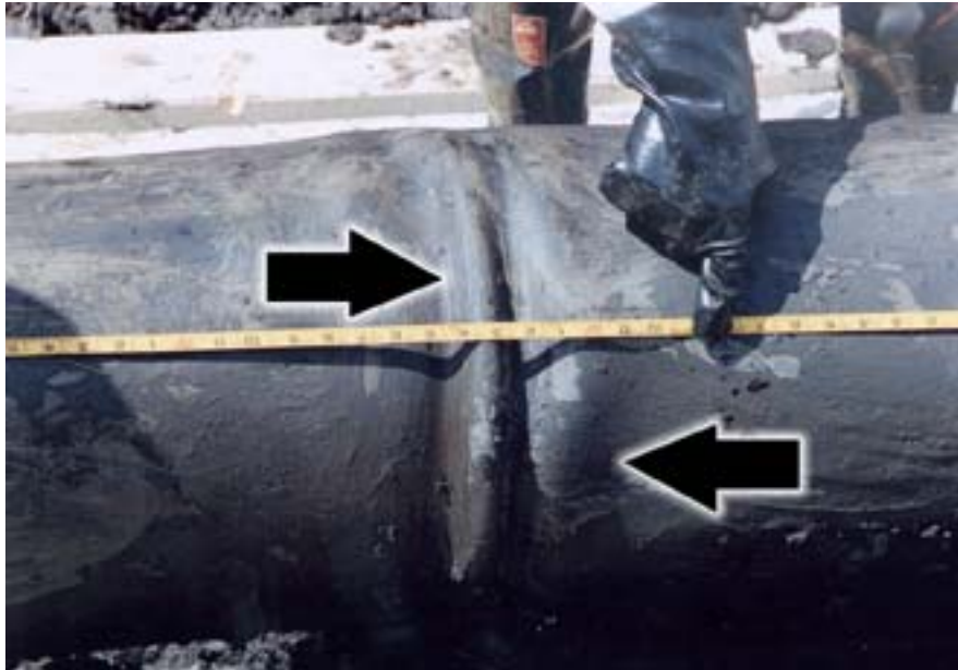
Figure 9. Indication of the buckle (Arrows show buckle location).
