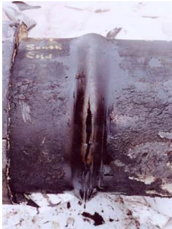
Figure 11. 6 1/2-inch-long, 3/8-inch-wide crack, with coating system shown at the left edge of photo.
