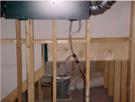
This is a properly trapped condensate tube.
