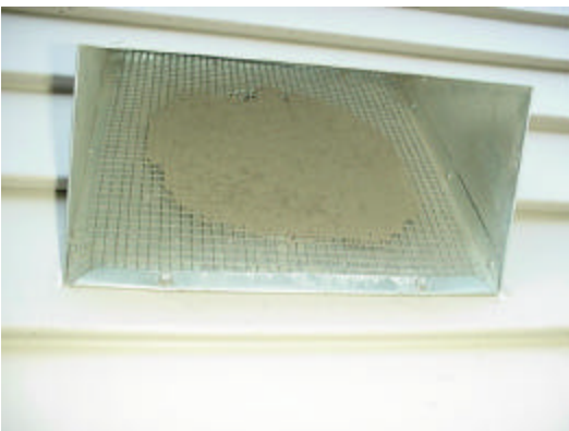
This is a typical plugged hood. Very little intake air is able to make it through the ¼” screen. The system will now have more exhaust capacity and could depressurize the structure.
