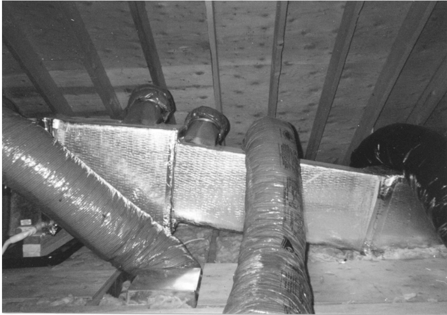
Figure 5-4 Mismatched Air Distribution System Components
