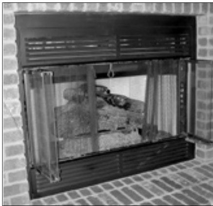
The flue, draft hood and outdoor air supply all contributed to leakage through atmospherically vented fireplaces.
