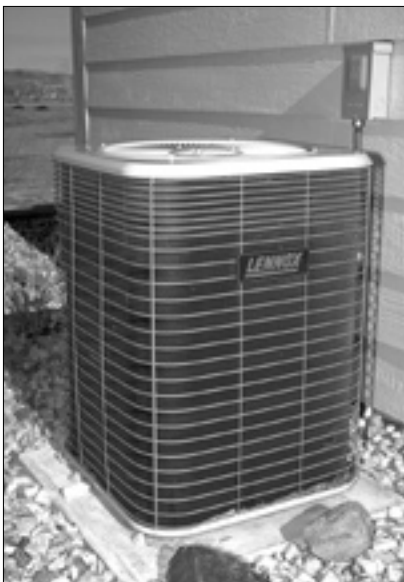
Outdoor air conditioning unit
