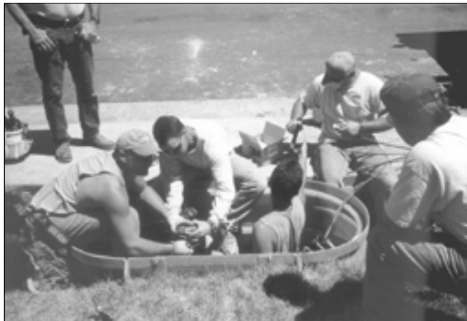
Fort Collins Utilities crew members change out a transformer that was overloaded under peak summer demand conditions.
