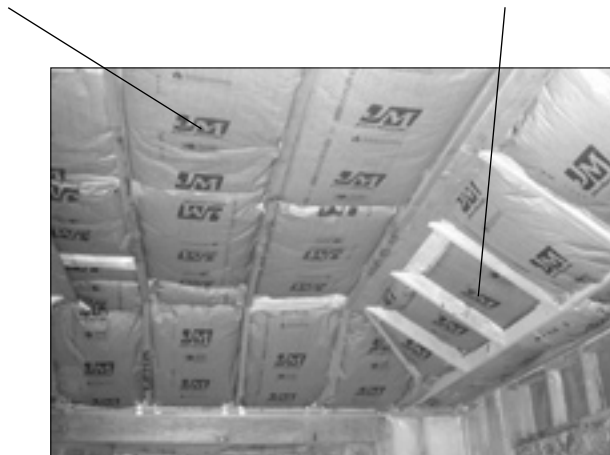
Vaulted and cathedral ceilings tended to have more insulation installation problems than flat ceilings.
