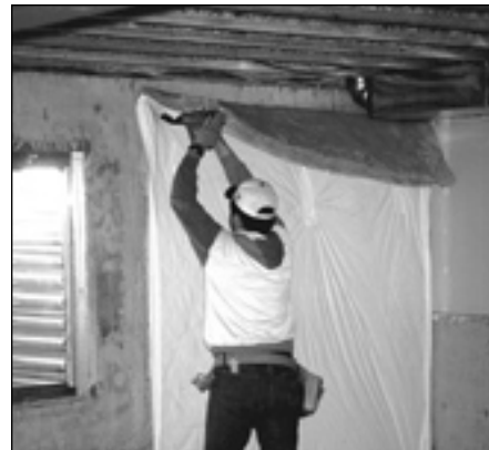
Basement wall insulation addressed one of the biggest remaining heat loss paths. The typical approach was a vinyl-faced fiberglass blanket on the interior of the concrete foundation.
