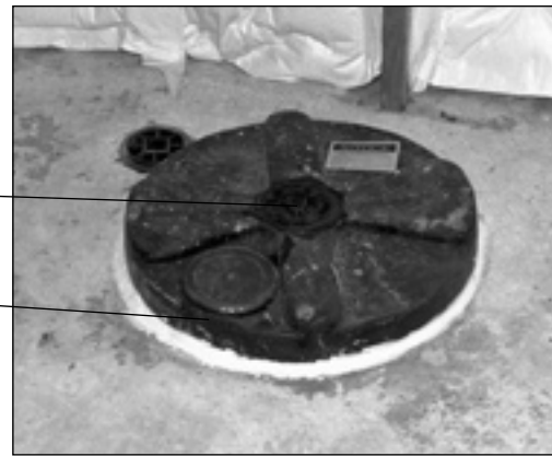
When air is drawn through an unsealed sump cover, it might bring with it radon, other soil gases or moisture.
