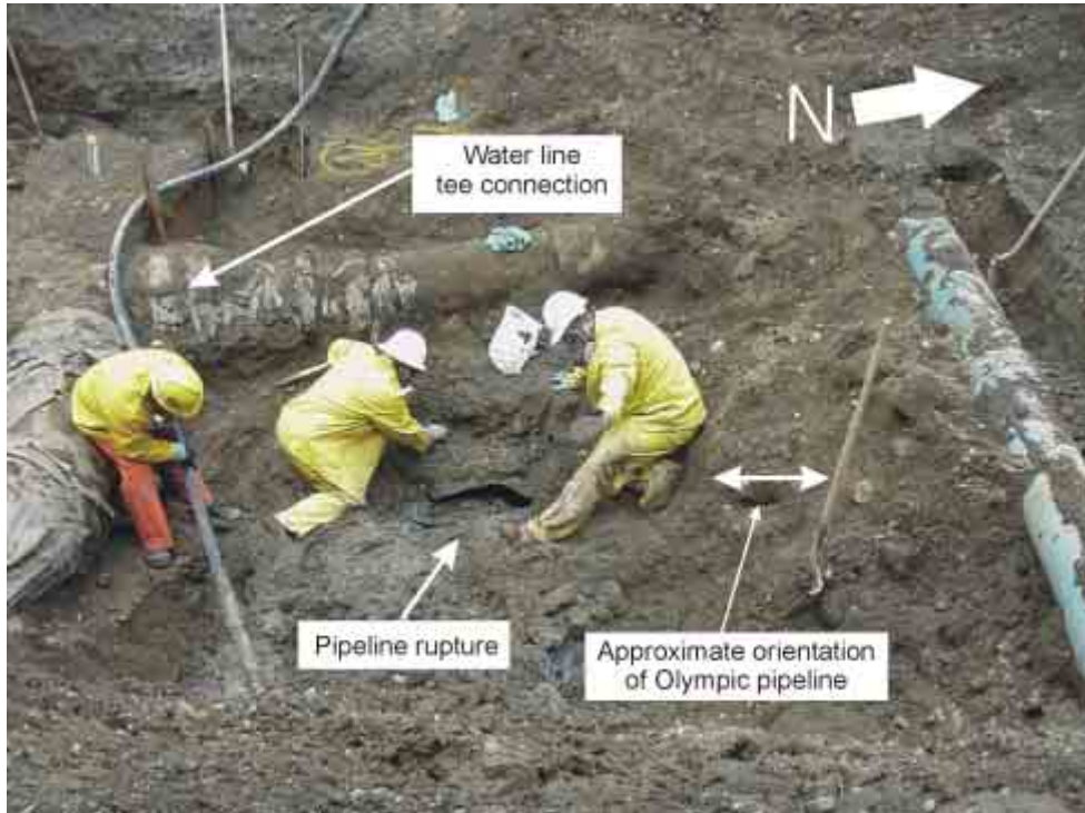
Figure 13. Rupture location before removal of pipe showing proximity of water line tee connection.
