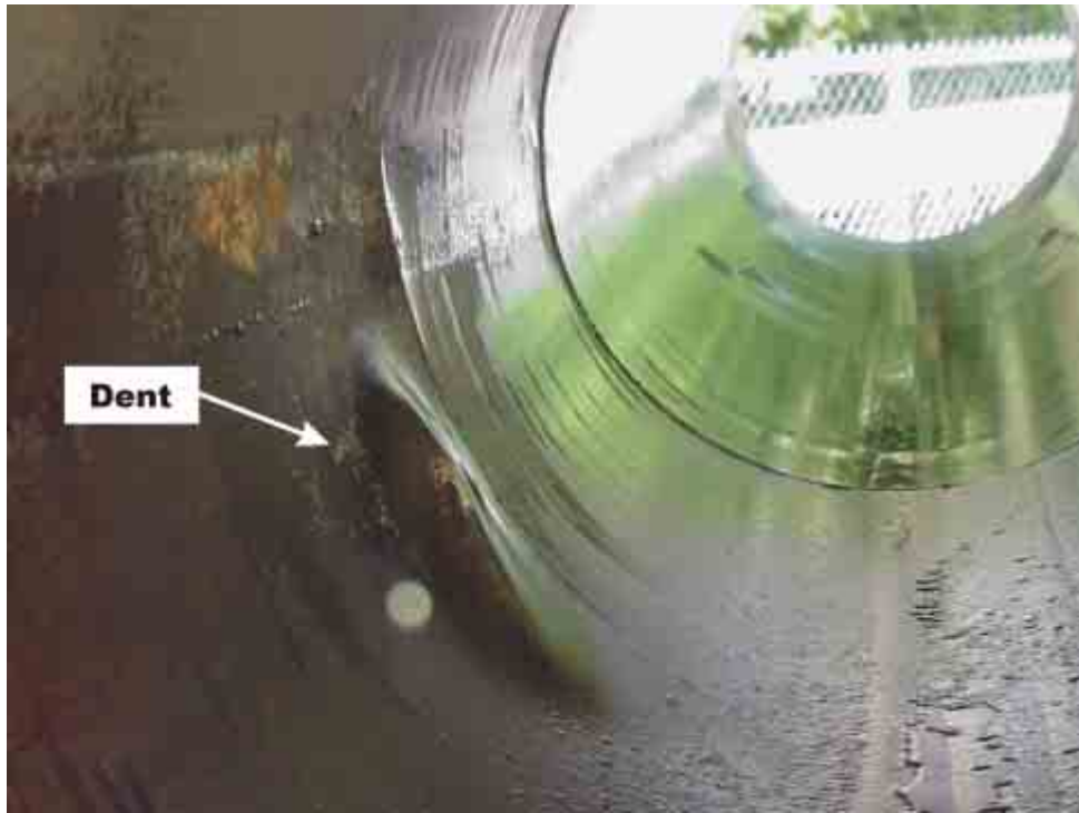
Figure 12. Inside view of second removed pipe section showing dent.
