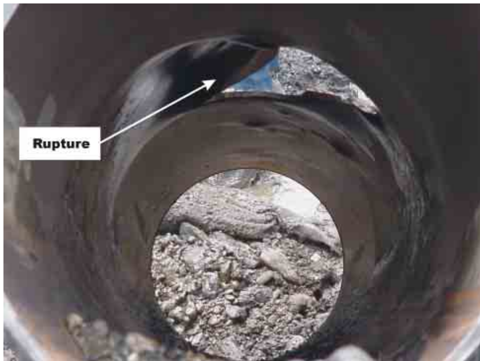
Figure 11. Inside view of ruptured pipe section.
