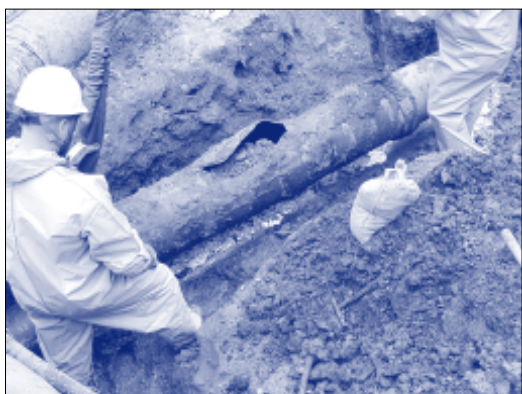
Investigator inspects pipeline rupture.
