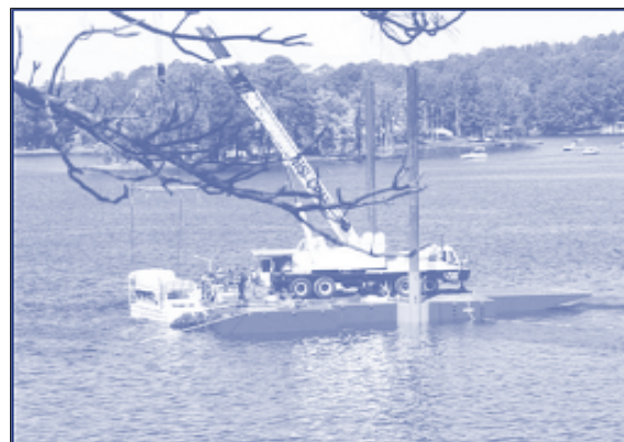
Salvage crew raises the M/V Miss Majestic from the bottom of lake.
