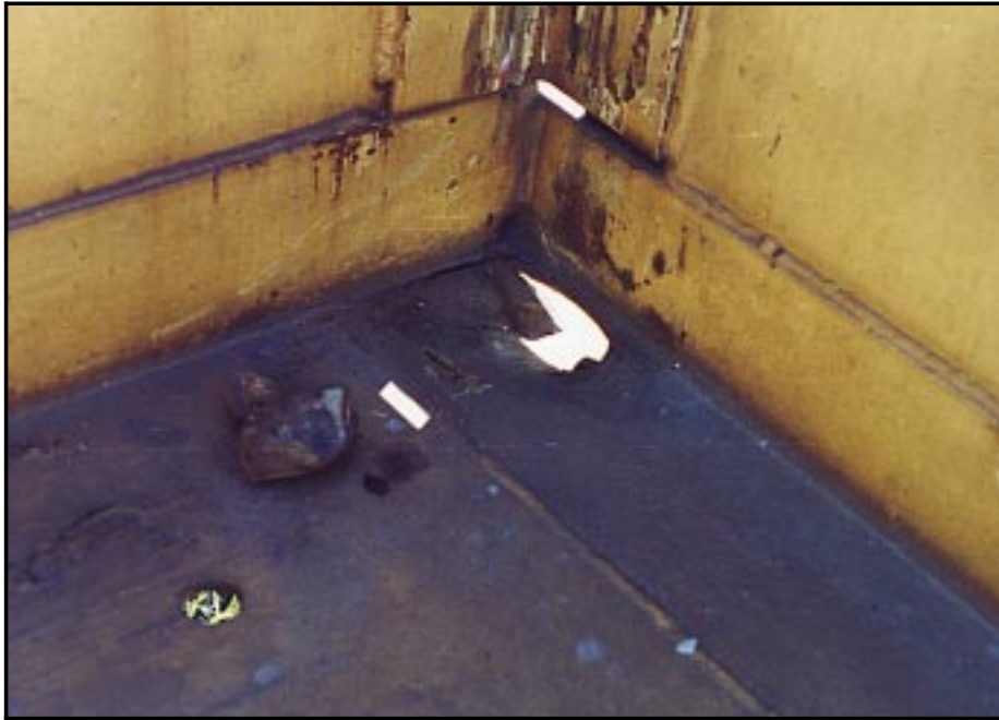
Figure 15. Damage caused by foreign objects to the platform floor of a Thrall double-stack car (two depressions and a hole). The larger depression (closer to hole) contains the imprint of a loose IBC.
