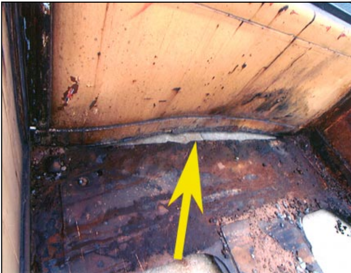
Figure 12. Gap as viewed from above car's platform
