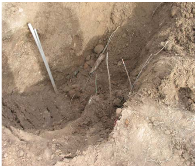
Buried Electrical Line Cut
