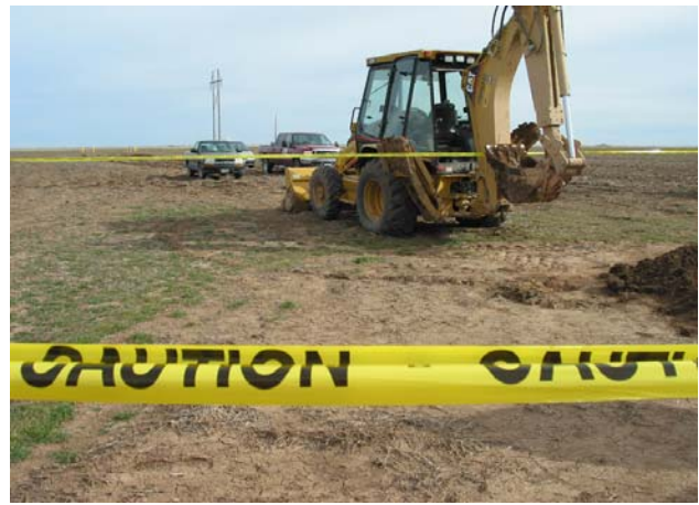
Excavation Event That Resulted in Cutting a Buried Electrical Line
