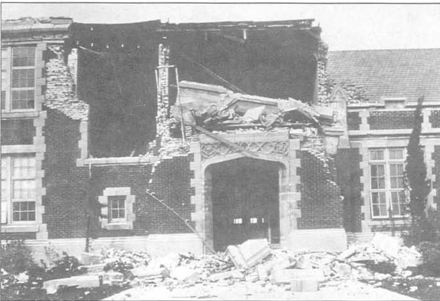
FIGURE B.2 This school building sustained severe damage in the 1933 Long Beach, California, quake. (Photo: U.S. Dept. of Commerce, NOAA)
