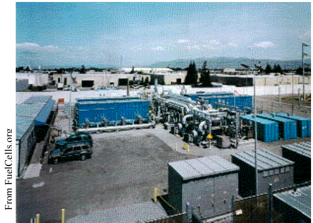
Figure 2-5. Fuel Cell Energy's 2 MW Molten Carbonate Fuel Cell power plant demonstration in Santa Clara, California
