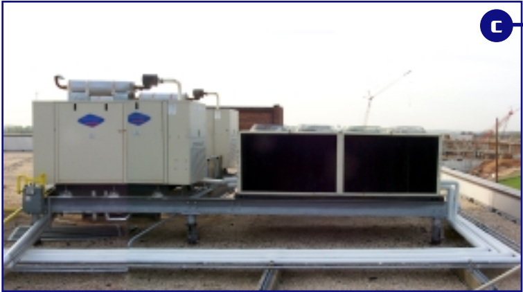
Engine-driven compressors and refrigerant condensers
