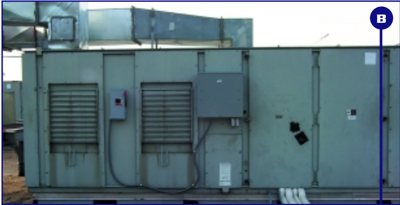
Rooftop air conditioning unit (RTU)
