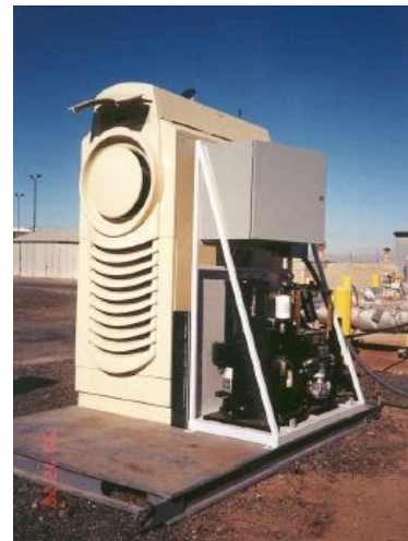
Figure 5-2: Landfill Gas Microturbine
