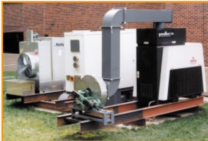
CHP Package System at the University of Maryland
