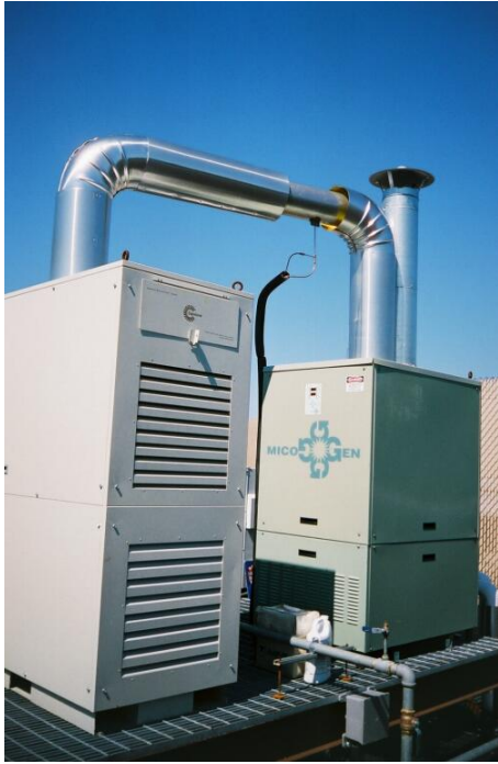
Figure 14: Roof-mounted DER Equipment (Microturbine and Heat Exchanger)
