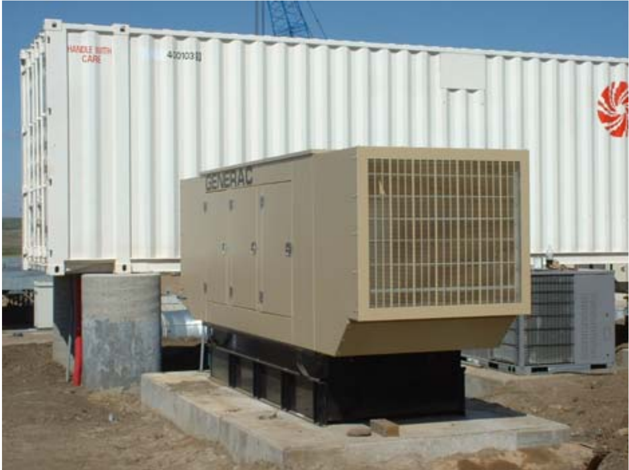
Figure 27. 225 kW Standby Generator On-Site For Emergency Backup ORMAT Modular Switchgear and Control Building in Background.
