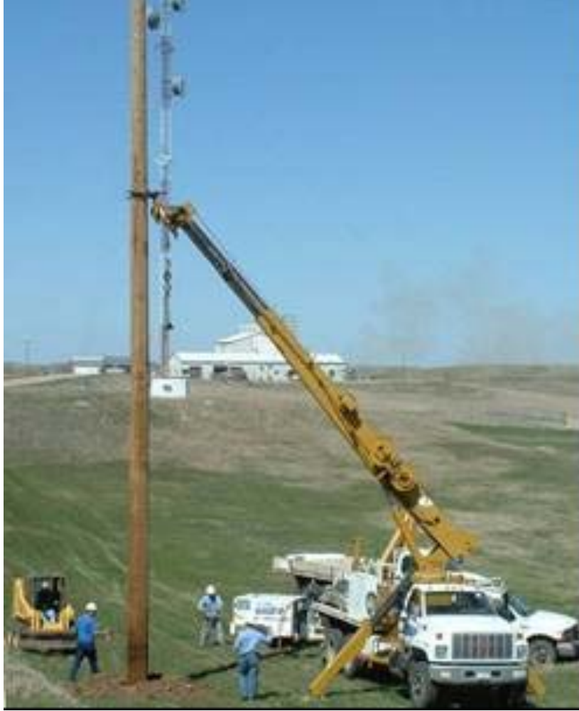
Figure 24. Feeder line from ORC to the Grid
