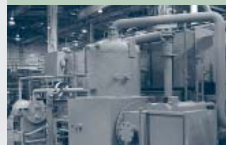
Triple Effect Chiller
