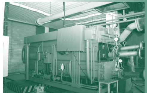
Lithium Bromide Chiller
