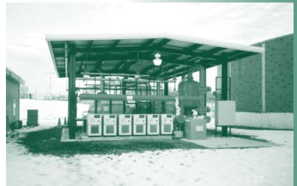
Pennsylvania Anaerobic Digester CHP System
