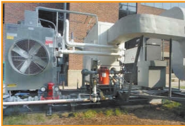
Microturbine, Exhaust Gas Fired Absorption Chiller, and Cooling Tower at the University of Maryland's IES for Buildings Integration Test Center
