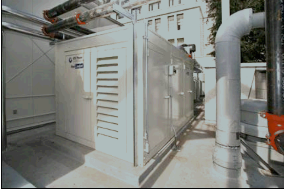
Figure 10 Installed Absorption Chiller with Enclosure
