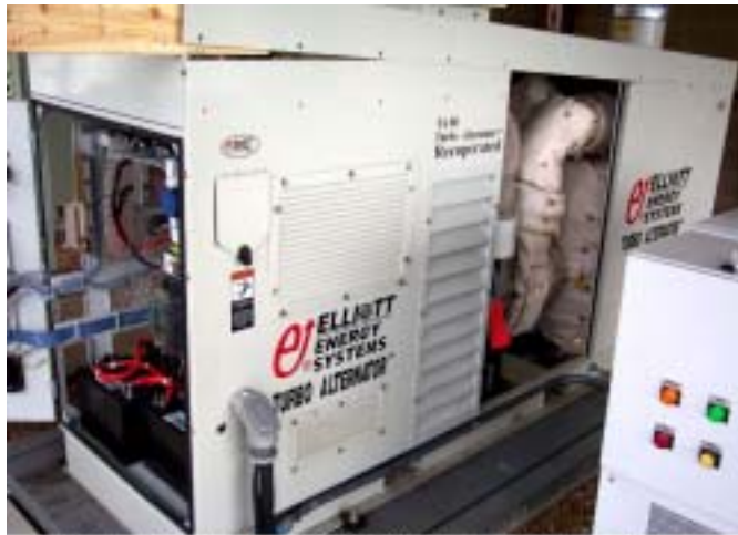
Elliott microturbine (80kW) opened for servicing
