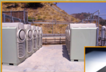
Capstone microturbine generators use air-cooled aluminum-finned heat sinks to cool the power electronics
