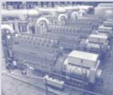
Internal combustion engines providing combined heat and power.
