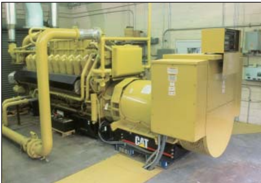
The U.S. Department of Energy has teamed up North America's three large gas engine manufacturers to implement the Advanced Reciprocating Engine Systems (ARES) program, which focuses on gas engine technologies to increase efficiencies, decrease emissions and lower life cycle costs. Caterpillar, with the introduction of its G3520C, has been the first to commercialize some of its ARES developments. Shown is a Cat G3520C gen-set installed in 2002 at Heber Light & Power in Heber City, Utah, U.S.A.
