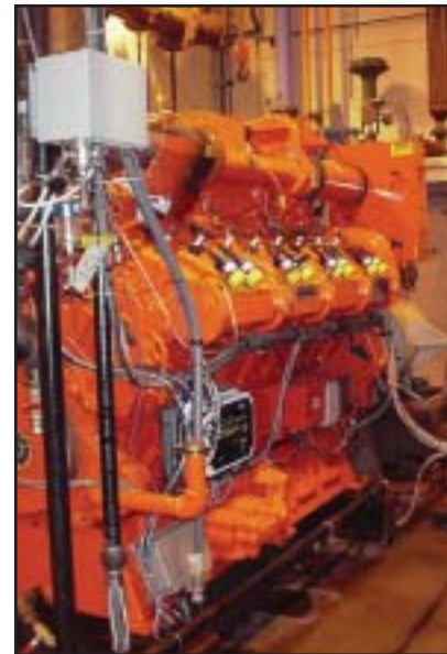
An instrumented Waukesha VGF engine with ESM controls at the company's test facility.
