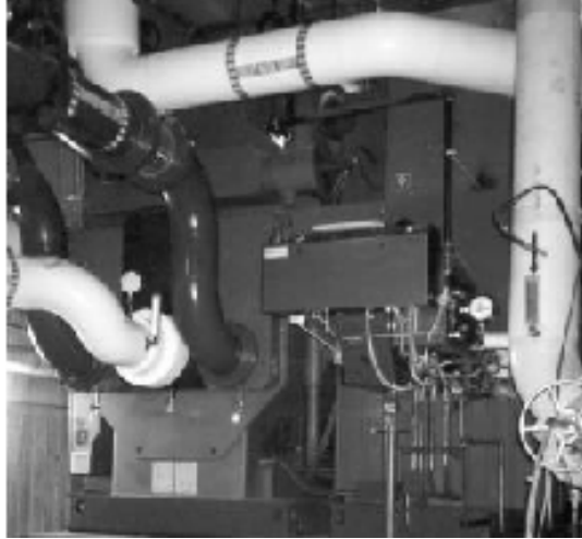
Figure 5. Direct-Fired Double-Effect Chiller/Heater Plant (523 Tons Chilled Water @44°F, 12 MMbtuh Hot Water @ 200 °F)
