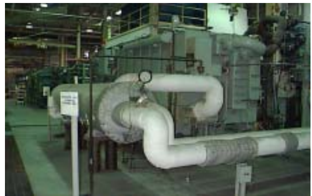
Figure 14: York Prototype Indirect-fired Triple-Effect Chiller
