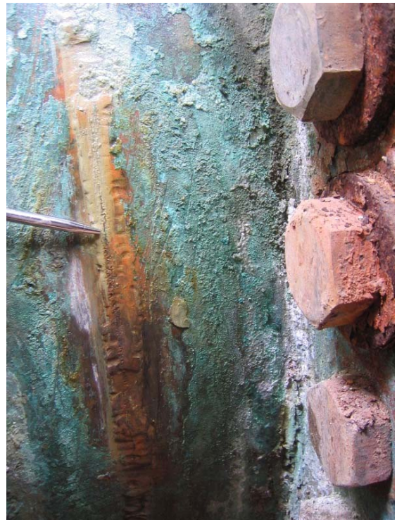
No. 12- Cracked weld in 54-inch pipe at Wye Vault at the MODE. Crack is the dark vertical line at the tip of the pen. Blue-green copper corrosion products covered the crack.
