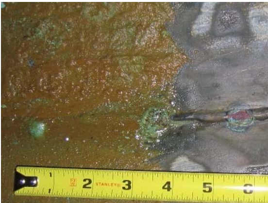
No. 14- Corrosion pitting on welds in bottom pipe shown in Photo No. 13. Pit at right has been cleaned to show reddish copper color from dealloying. Mound of blue-green corrosion product at left is underlain with the same type of pit.
