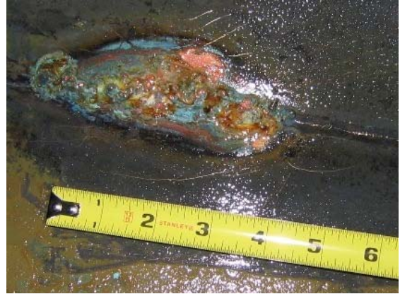
No. 15- Close view of repair weld found under mound of corrosion products in foreground of Photo No. 13. This location is on along the longitudinal weld at the bottom of the pipe.
