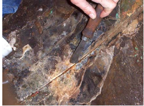
No. 11- Unwelded joint in the 72-inch header pipe at the Intake Pumping Station. This location was found covered with silt, suggesting that groundwater leaked into the pipe through this joint.
