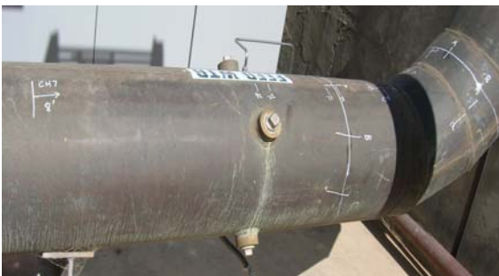
No. 1- Aluminum bronze pipe test section CH-7. White marks at right indicate bands of ultrasonic thickness test points.
