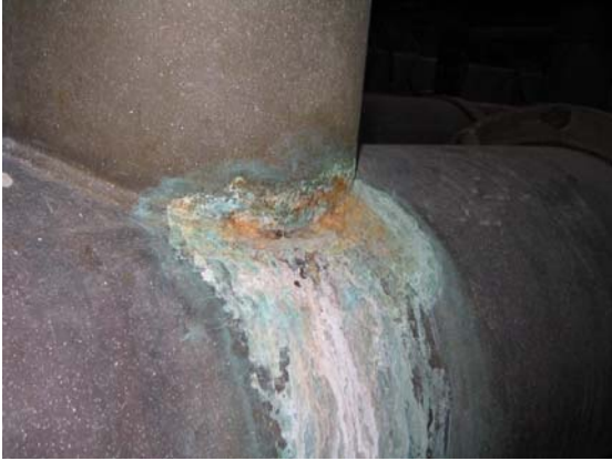
No. 9- Seeping leak at original weld in aluminum bronze pipe in Desalting Building.
