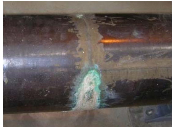
No. 8- Seeping leak at repair weld in aluminum bronze pipe in Desalting Building.
