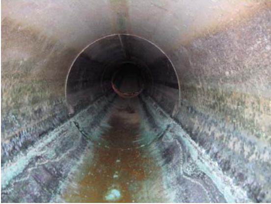
No. 13- Interior of 30-inch Hydranautics Feed pipe at location CH-19. Blue-green corrosion products are evident below the water line on the longitudinal weld (foreground) and on the circumferential weld (center).
