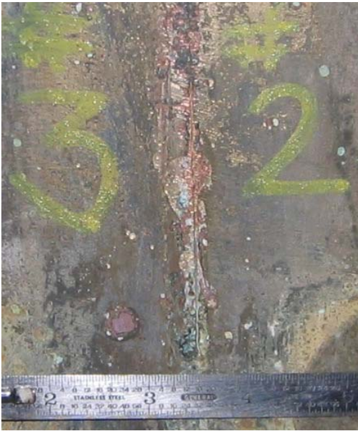
No. 10- Typical cracked circumferential weld in 72-inch header at Intake Pumping Station. The crack is the vertical line from above the ruler. This crack is in the weld between pipe piece nos. 2 and 3.
