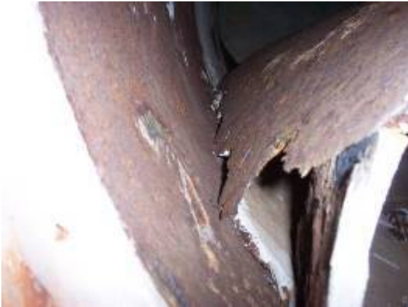
Spalling of Concrete Pipe Lining
