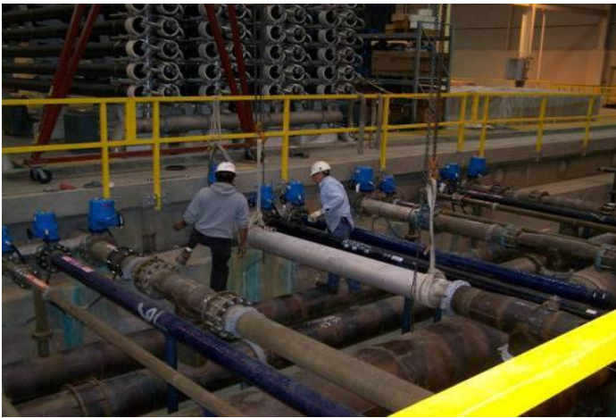
Bright Blue Devices are Control Valves and Actuators
