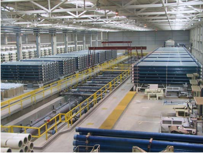
Hydranautics Desalting Vessels
