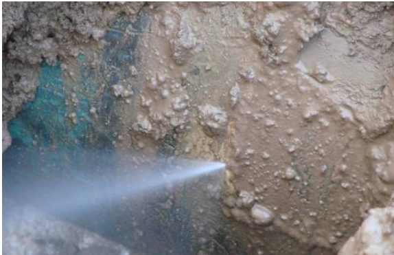
Leak in Aluminum-Bronze Pipe during Demonstration Operation
