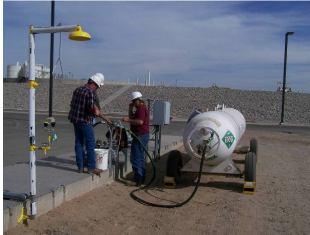
Temporary Ammonia Injection System
