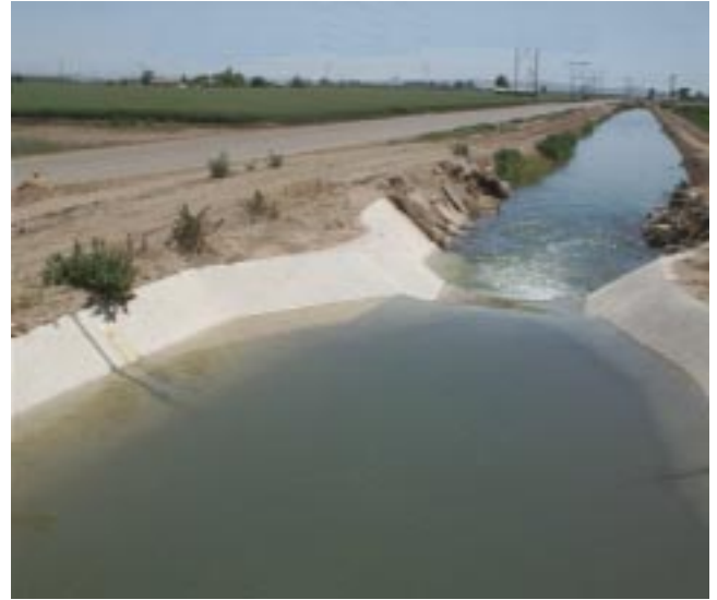
Long Throated Flume in Earthen Canal
