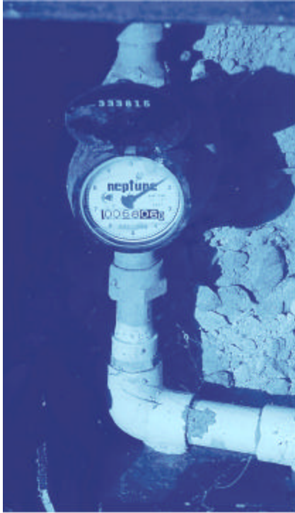
Photo 2. Residential water meter
