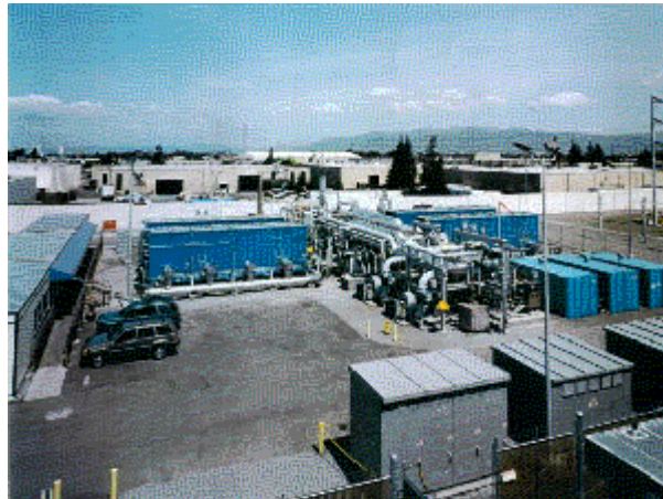
Figure 2-9. Fuel Cell Energy's 2MW Molten Carbonate Fuel Cell power plant demonstration in Santa Clara, California
