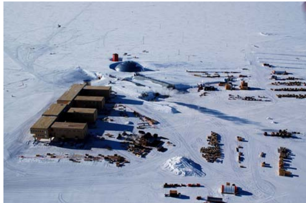
Progress continues on the new U.S. research station at the South Pole. This season marked completion of all steel and panel enclosure work for all wings. On January 30, 2005, the project accepted for conditional occupancy the wings for housing, science space, and emergency power. Credit: USAP
